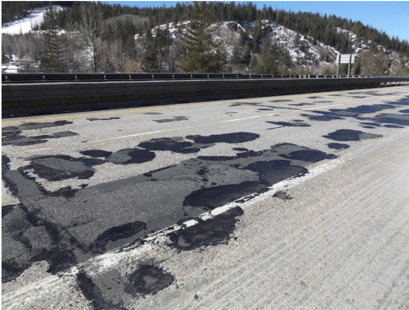
Figure 5-23: Example of Poor Condition Bridge Deck
