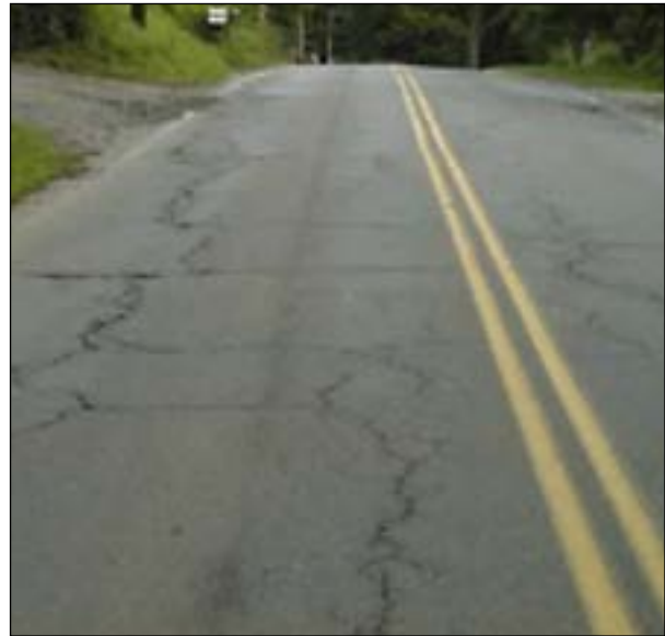
Exhibit 2-11: Block and Longitudinal Cracking
