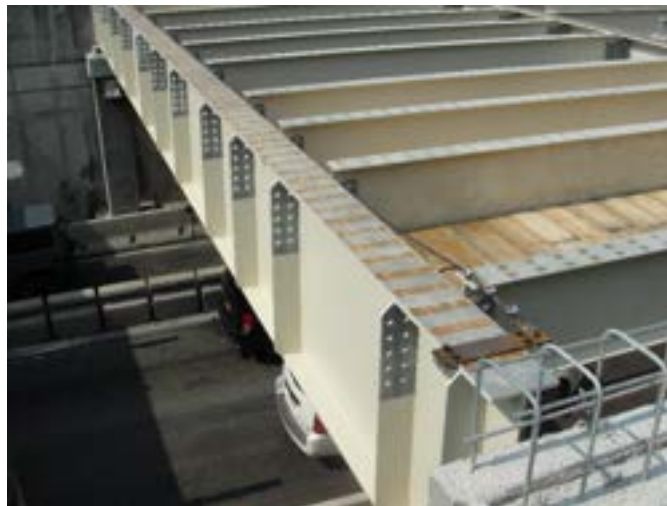
Source: Gannett Fleming Photo - NJ Route 139 Reconstruction.
