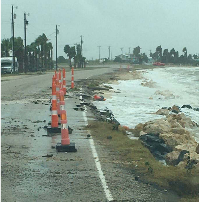
Figure 5-15. State Highway 316 Storm Damage
