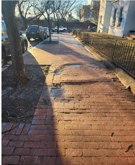
Brick Sidewalk – damage by tree roots
