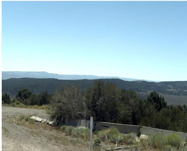
Figure 42. GEMMA CASE #2, Image of a Spalled Precast Concrete Barrier
