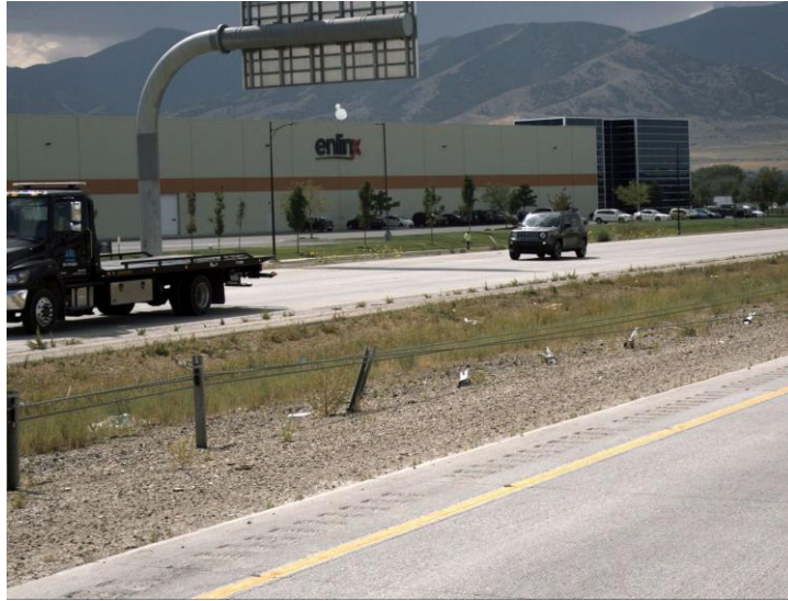
Figure 32. Llama CASE #4, Image of Broken Cable Barrier Posts along a Road
