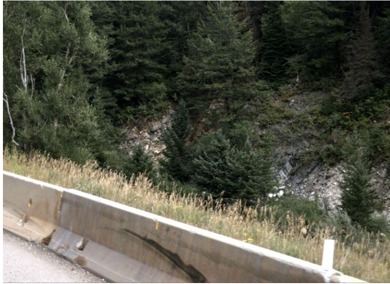
Figure 34. Llama CASE #6, Mountain View and Concrete Barriers
