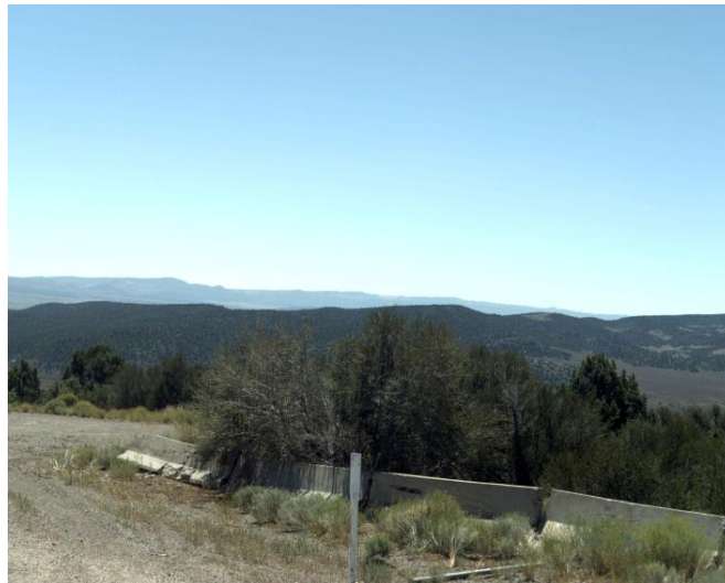
Figure 22. QWEN CASE #1, Image of a Spalled Precast Concrete Barrier
