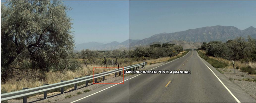
Figure 6. Example of an Annotated Image with a Missing/Broken Post
