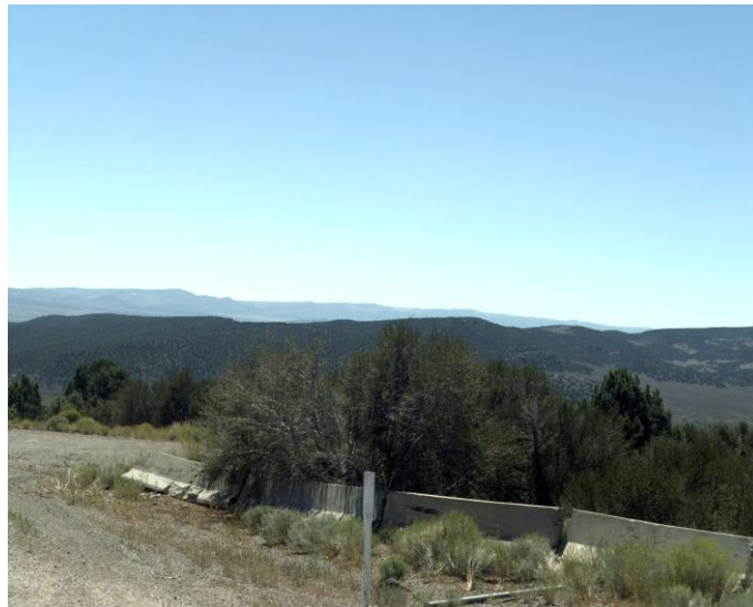
Figure 23. QWEN CASE #2, Image of a Spalled Precast Concrete Barrier
