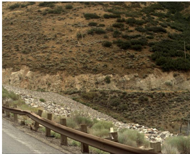
Figure 30. Llama CASE #2, Image of a Deflected Guardrail
