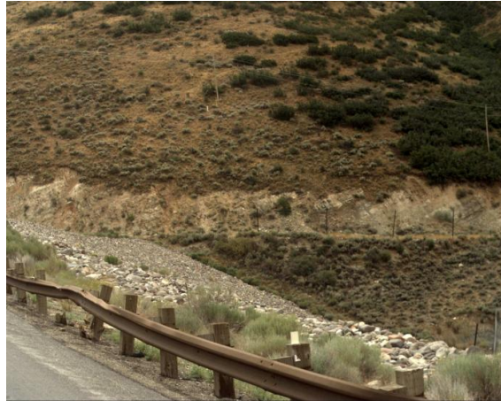
Figure 41. GEMMA CASE #1, Image of a Deflected Guardrail
