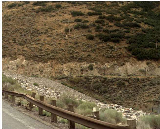
Figure 29. Llama CASE #1, Image of a Deflected Guardrail
